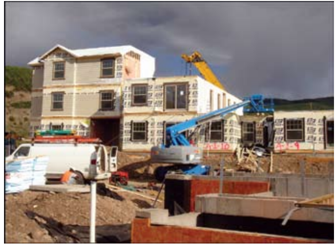
The Club Commons II was completely set in only 12 days. In addition to rapid set times modular construction resulted in minimal materials waste during construction.
