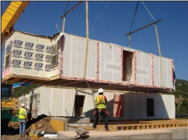
A modular section from Barvista Building Systems is lowered by crane on the second day of assembly. The entire project is LEED (Leadership in Energy and Environmental Design) certified.
